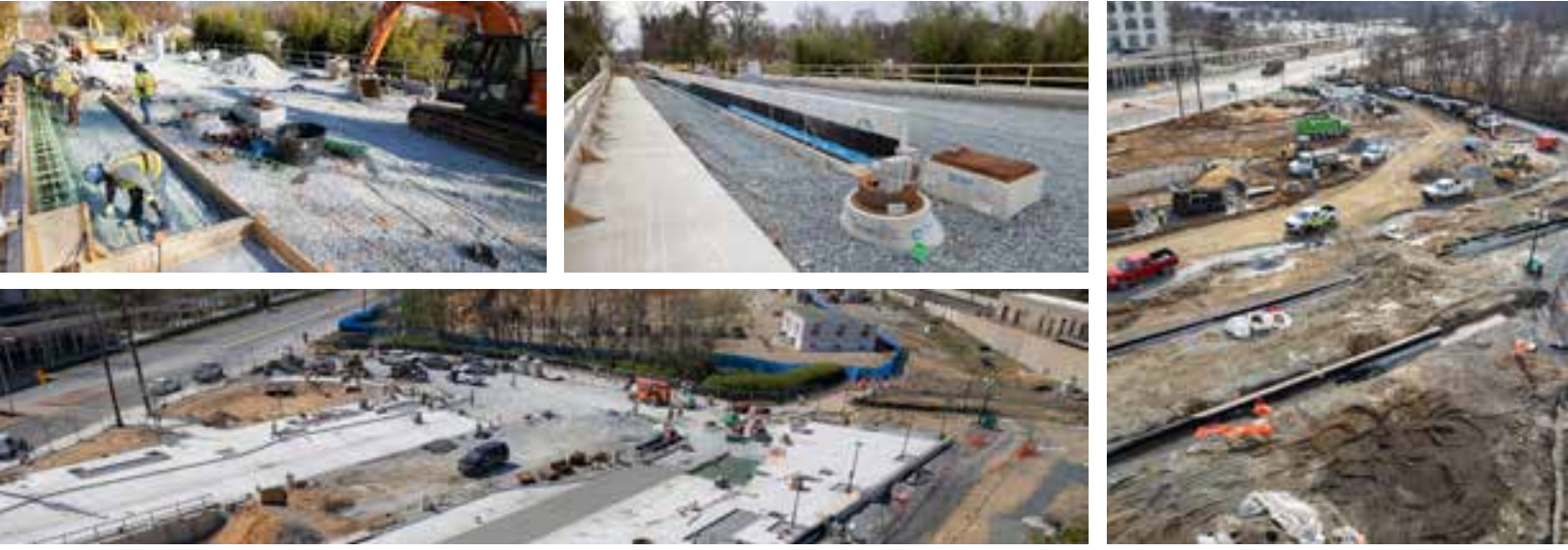
Photos clockwise from left: Crews from Terra Site Constructors work on the Sleaford Road overpass in Bethesda in December; Work progresses with the goal of opening the underpass this summer; Crews from Priority Construction work to build the College Park Metro Bus Loop; The bus loop is taking shape in this photo from last Friday.
